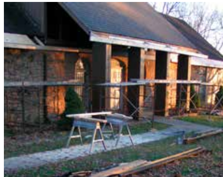
In November the roof and gutters of the Shrine were repaired and the roof of the residence was also repaired. In November repairs to
